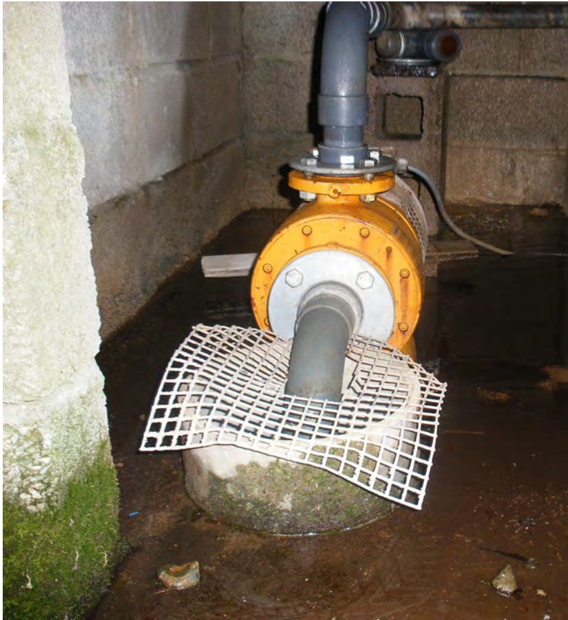
Figure 8 – Borehole pump at Houghton Springs Fish Farm.
